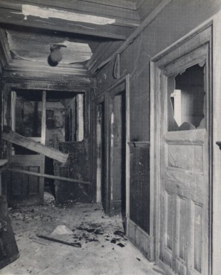
The 5th floor doors were badly burned.
